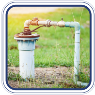
Ground Water Metering
